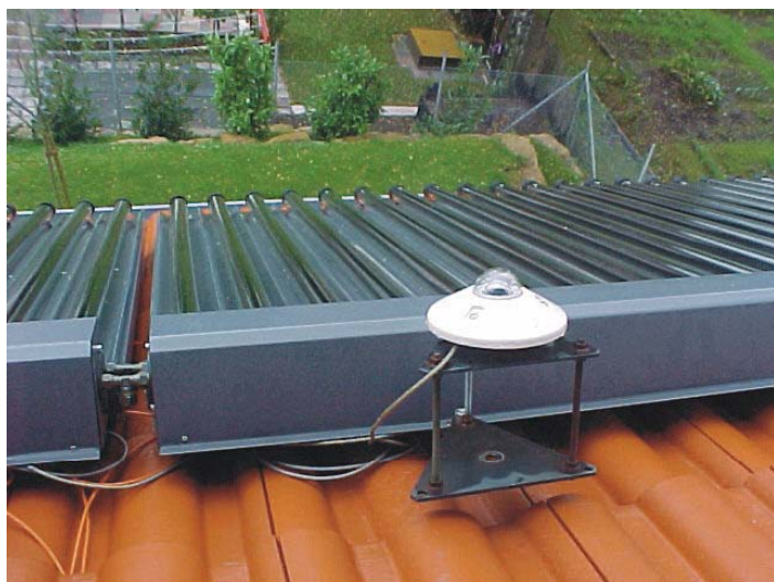
Figure 1: View of the collector field.
