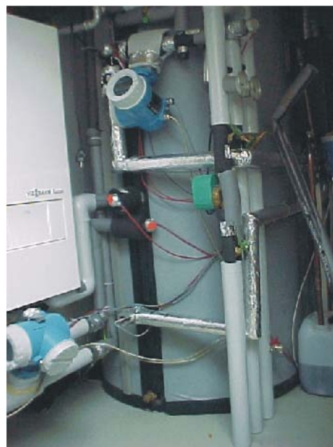
Figure 2: Storage with measurement equipment
